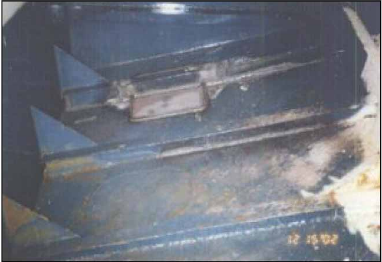
Figure 21: Photograph taken inside of potable water tank showing doubler.
