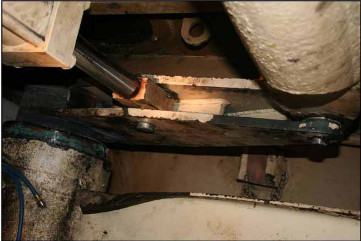
Figure 30: Steel Tiller Assembly showing hydraulic steering system connection and cross connect (from M/V DEFENDER)
